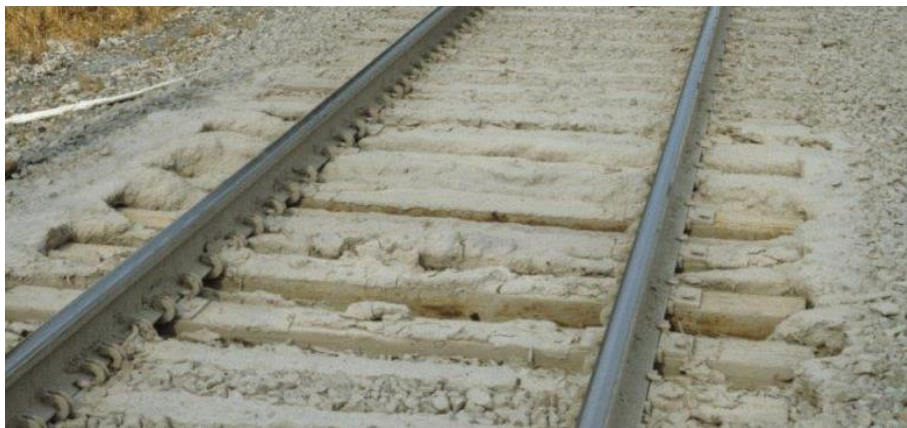
Figure 7. Ballast with Slurry-Formed Voids Under and Around Ties After Ballast Life Has Expired
