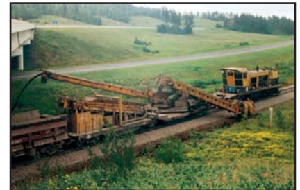
Conveyor. The Badger's conveyor system discharges material on either side of the track or into an air dump car towed behind.
