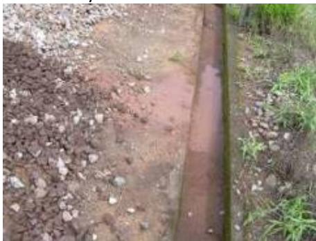
Fig. 7. Fine material carried down by rain water Bom Jardim – MG
