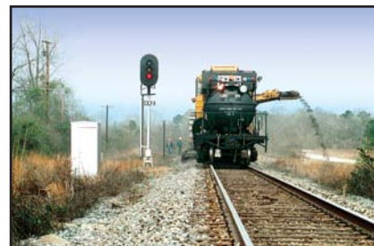
Ballast discharge. The HP distributes the cleaned ballast along the shoulders, at a rate that can be varied for local conditions. Plus, it establishes the railroad specified shoulder slope as it works at speeds of up to 2 mph (3.2 kph).
