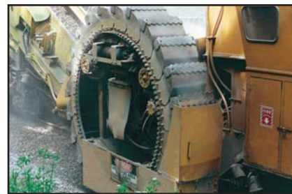
Digging wheel. Two digging wheels rip through compacted ballast to a depth of up to 16 inches (400 mm) from the top of the tie. Each wheel is 30 inches (760 mm) wide to allow cleaning from the ends of the ties to the edge of the shoulder.
