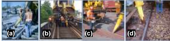
Figure 14: (a) Undercutting Switch, (b) Undercutting Bridge Deck, (c) Debris Cleanup, (d) Bridge Deck Cleaning
