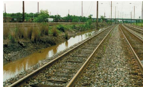
Standing Water In Ditch
