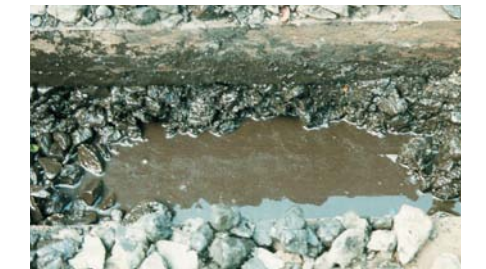
Water Trapped In The Track
