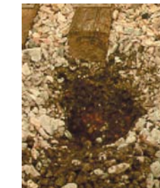
Contaminated Ballast Shoulder
